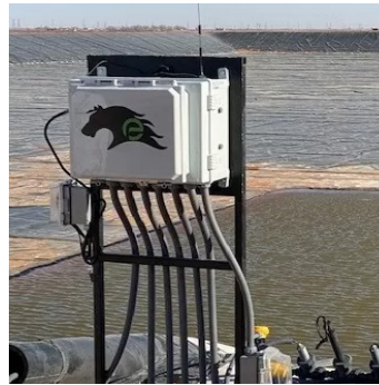
Remote Water Monitoring System
