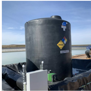
Automated Chemical Injection
